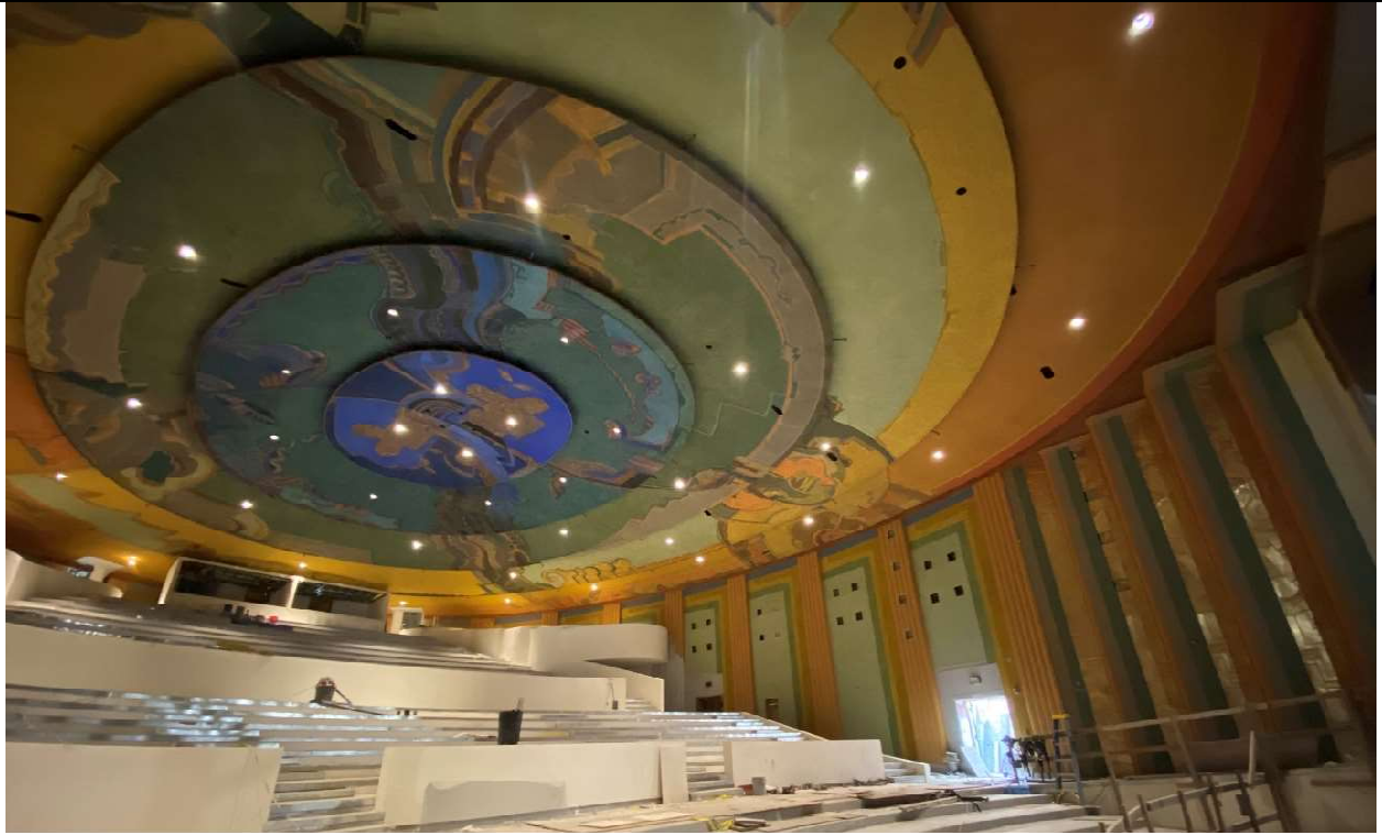
Interior view of the Vision Theatre audience chamber & historic ceiling (restoration in-progress)
