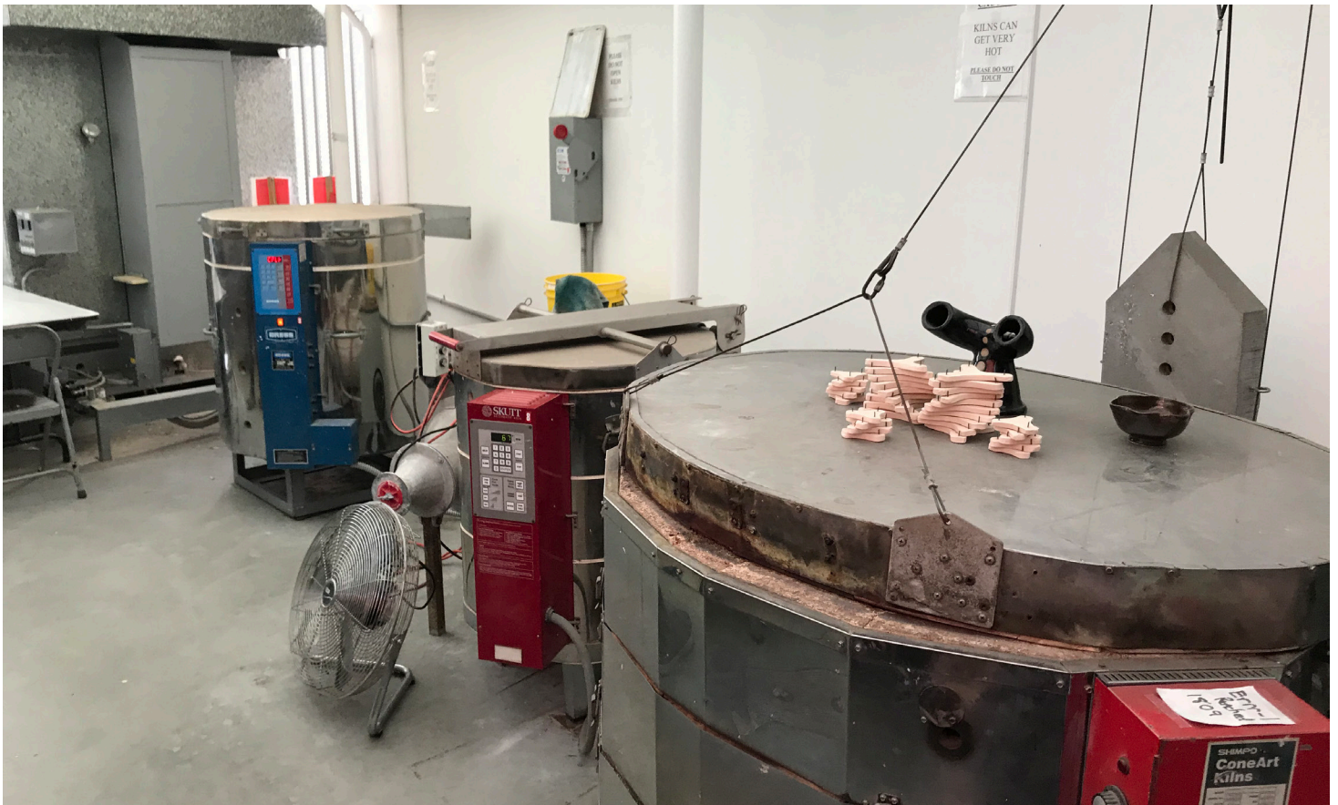
▲ Kiln Room - A dedicated room adjacent to the pottery studio house the kilns, providing the necessary electrical connections and ventilation.
