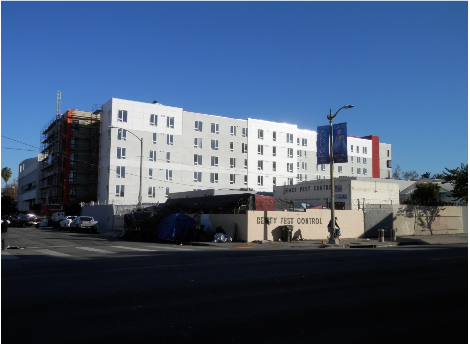
Path Metro Phase 2. View of site at corner of Beverly Blvd & Madison Ave.
