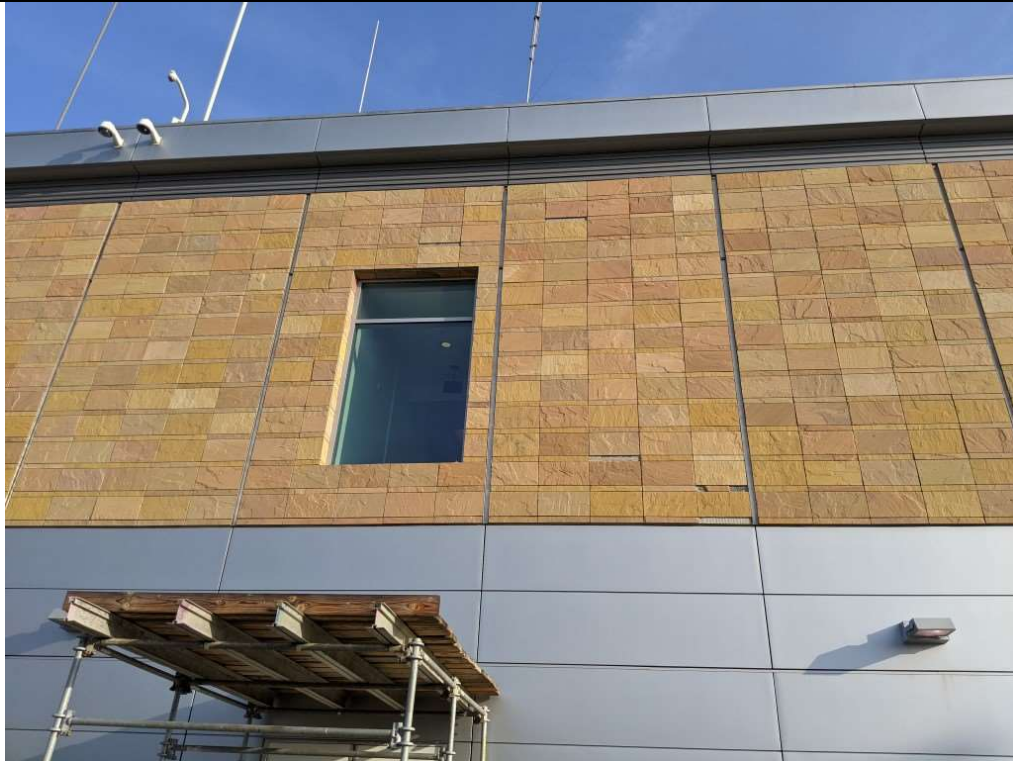
Erected scaffolding over entrance on South Side. Visible tiles fallen from façade
