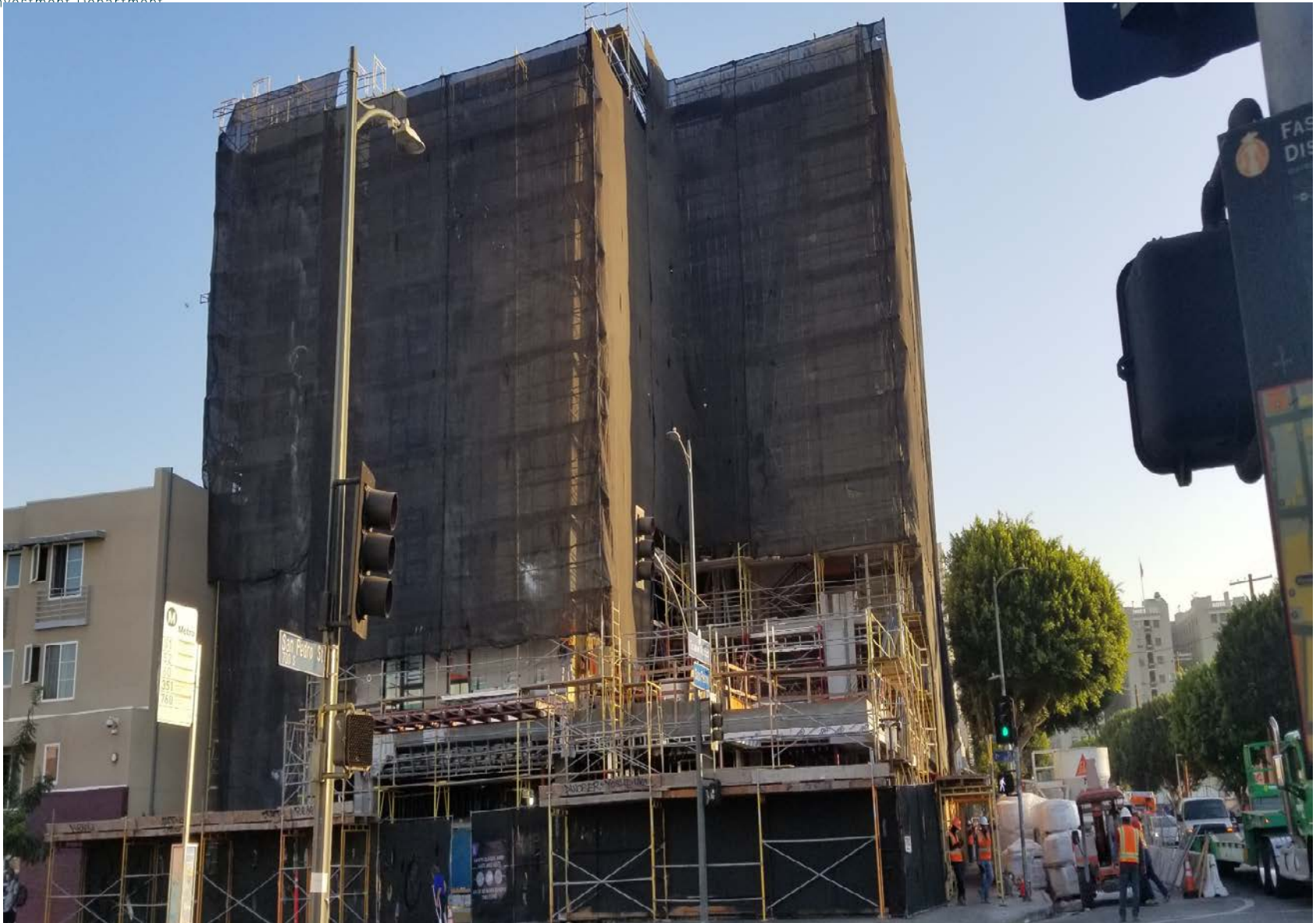
Located at 519 E 7 th St. View from across the intersection on 7 th & San Pedro St.
