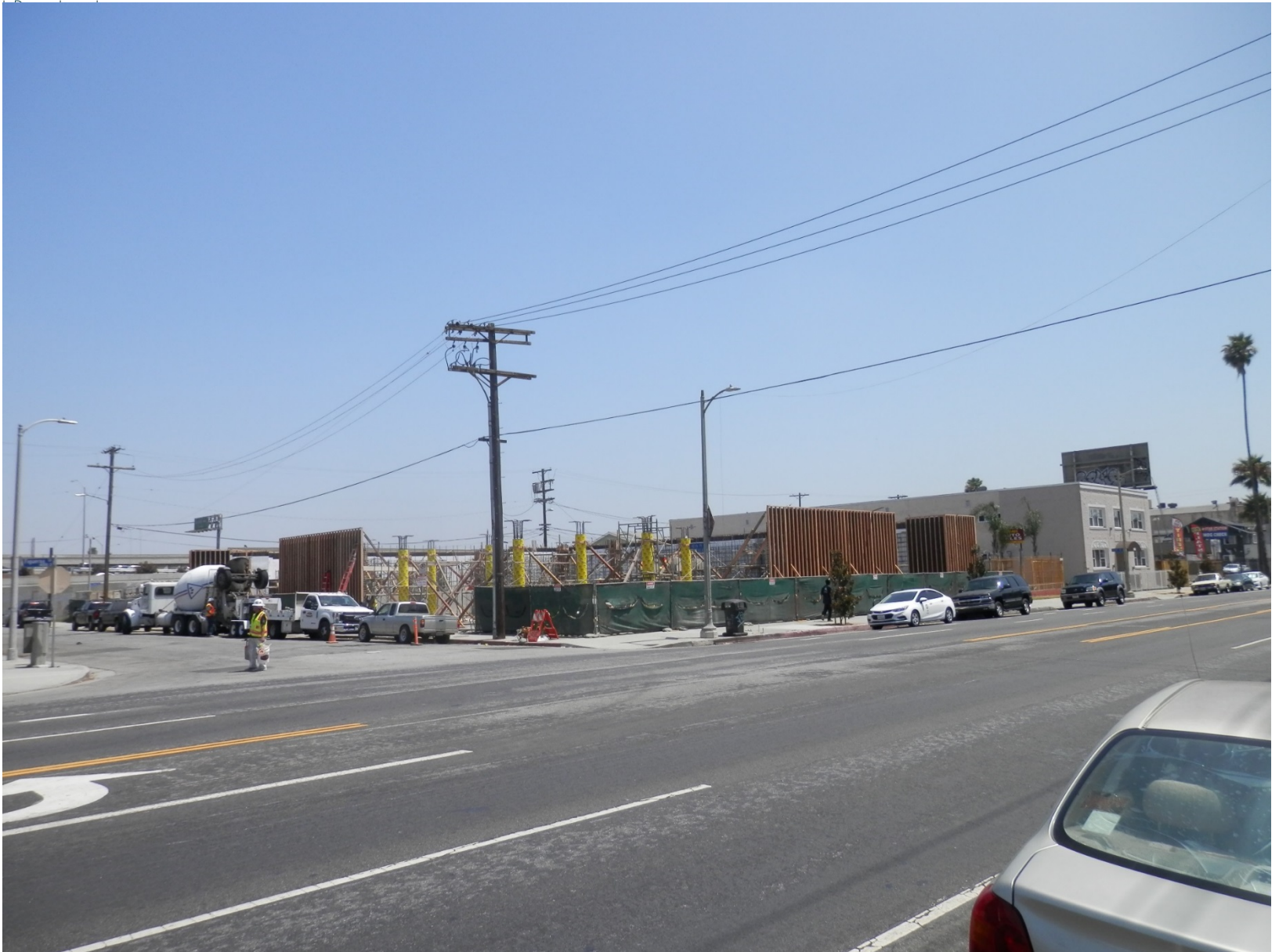
Located at 4050-60 S. Figueroa St. View from just inside fence on 40 th Pl.
