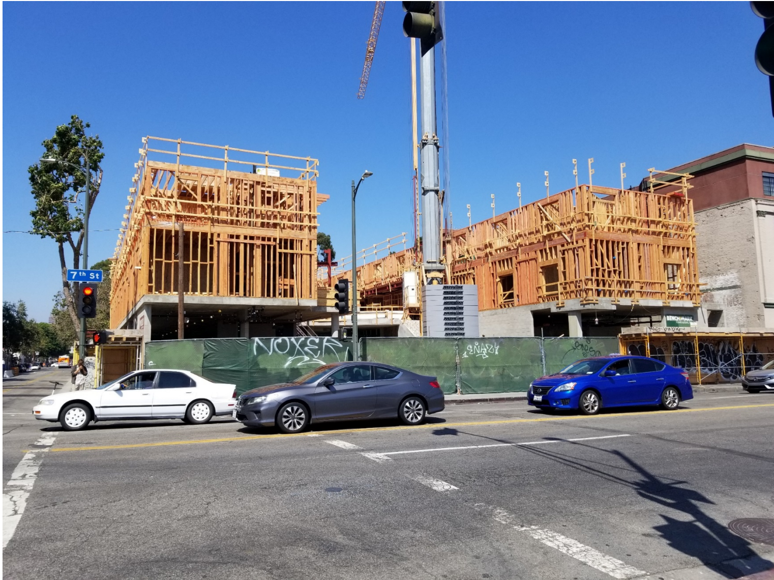
Located at 401 E 7 th St. . View from third floor of 649 lofts across Wall St .
