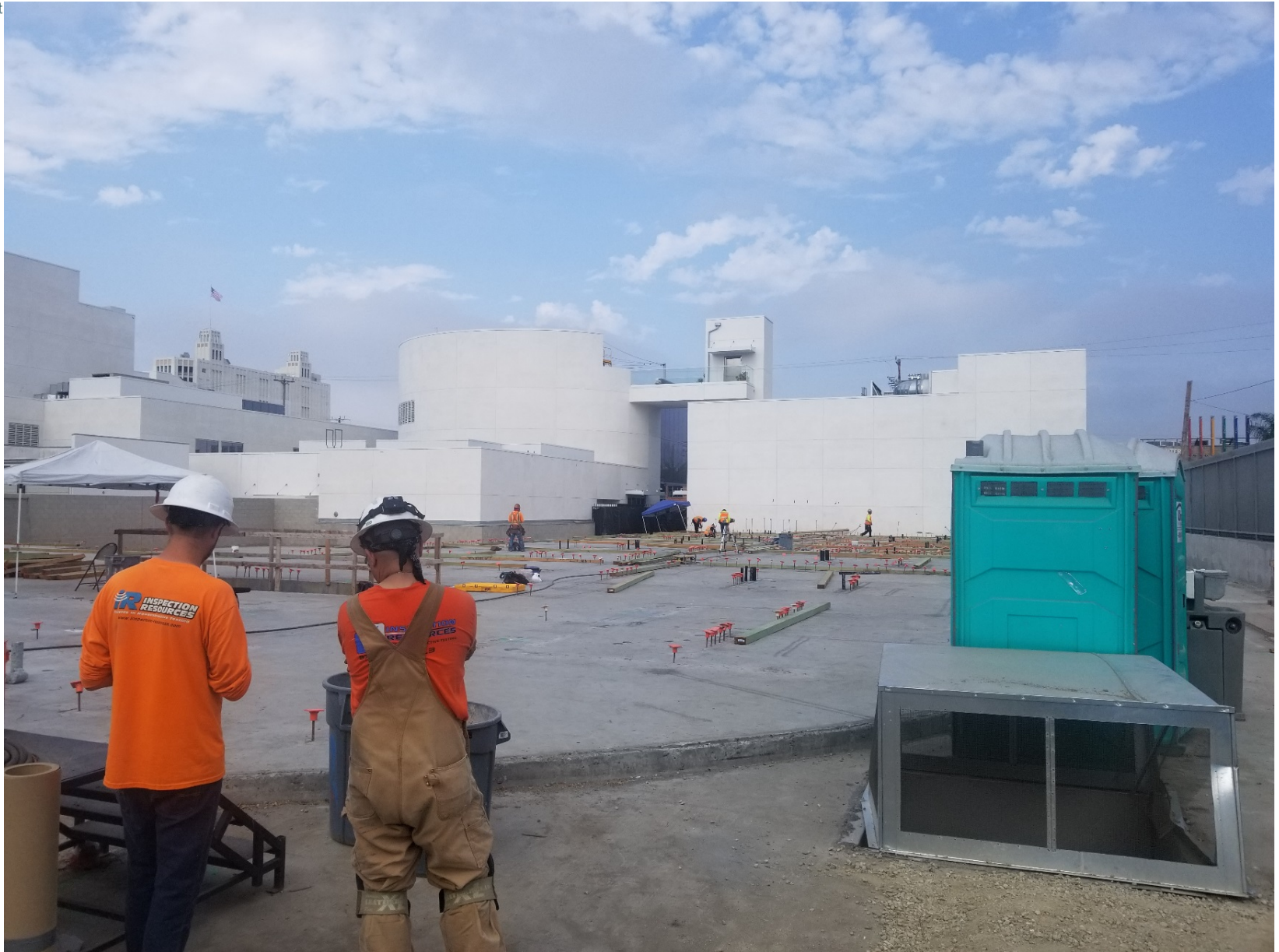
Located at 1119 N. Mc Cadden Pl. . View from just inside of fence of situs.
