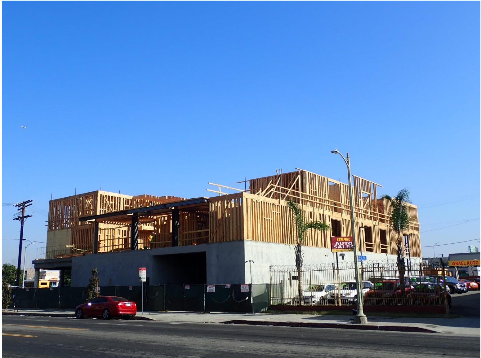
Located at 4050-60 S. Figueroa St. View from across the street of site.
