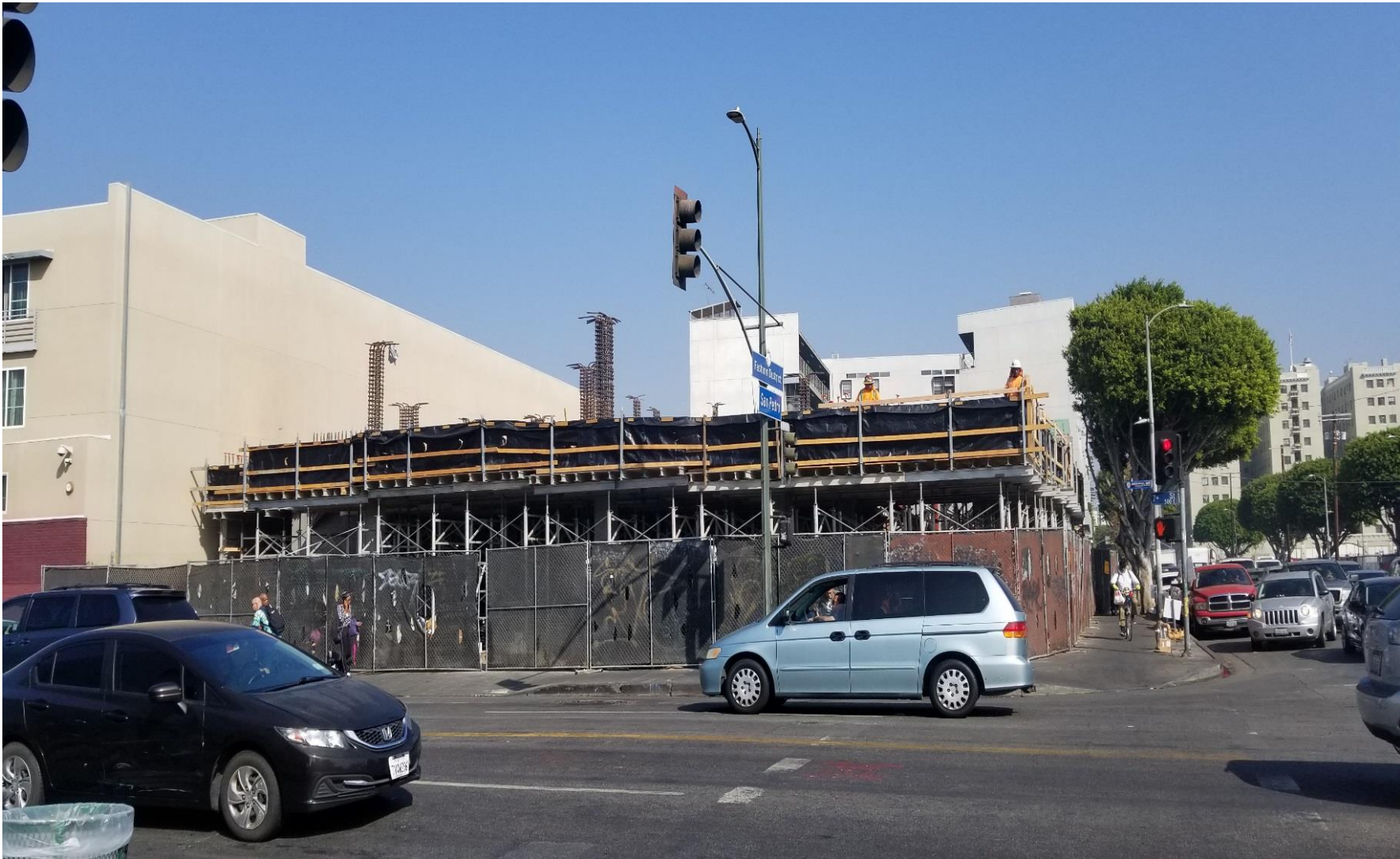
Located at 519 E 7 th St. View from across the street on 7 th St.
