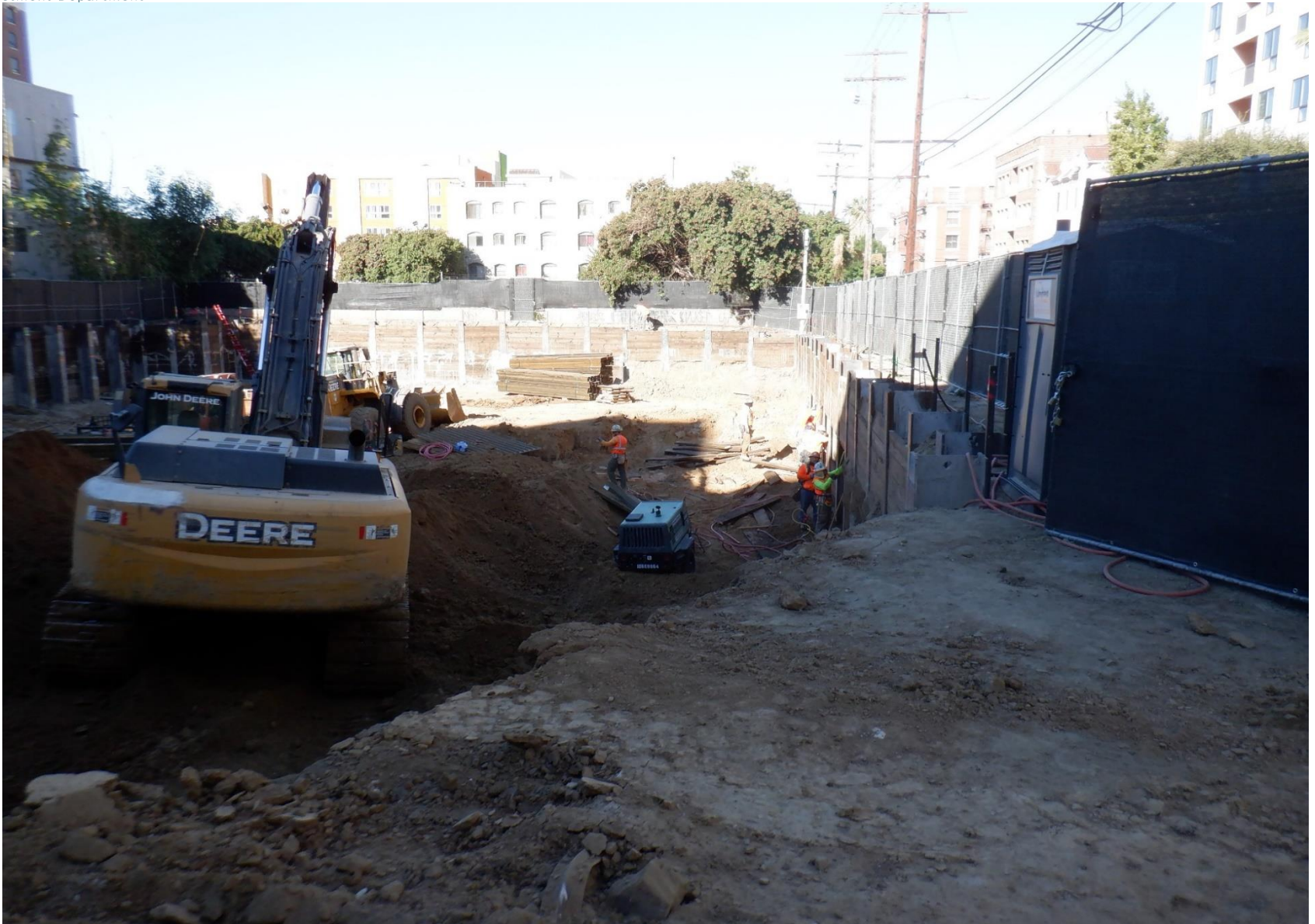
View from inside the fence at 1218 Ingraham St.
