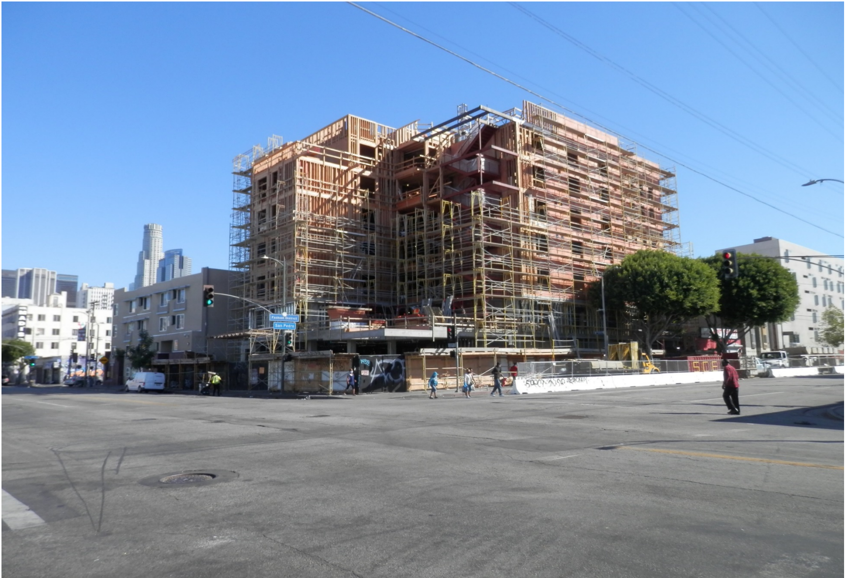
Located at 519 E 7 th St. View from inside the construction fence on 7 th St.
