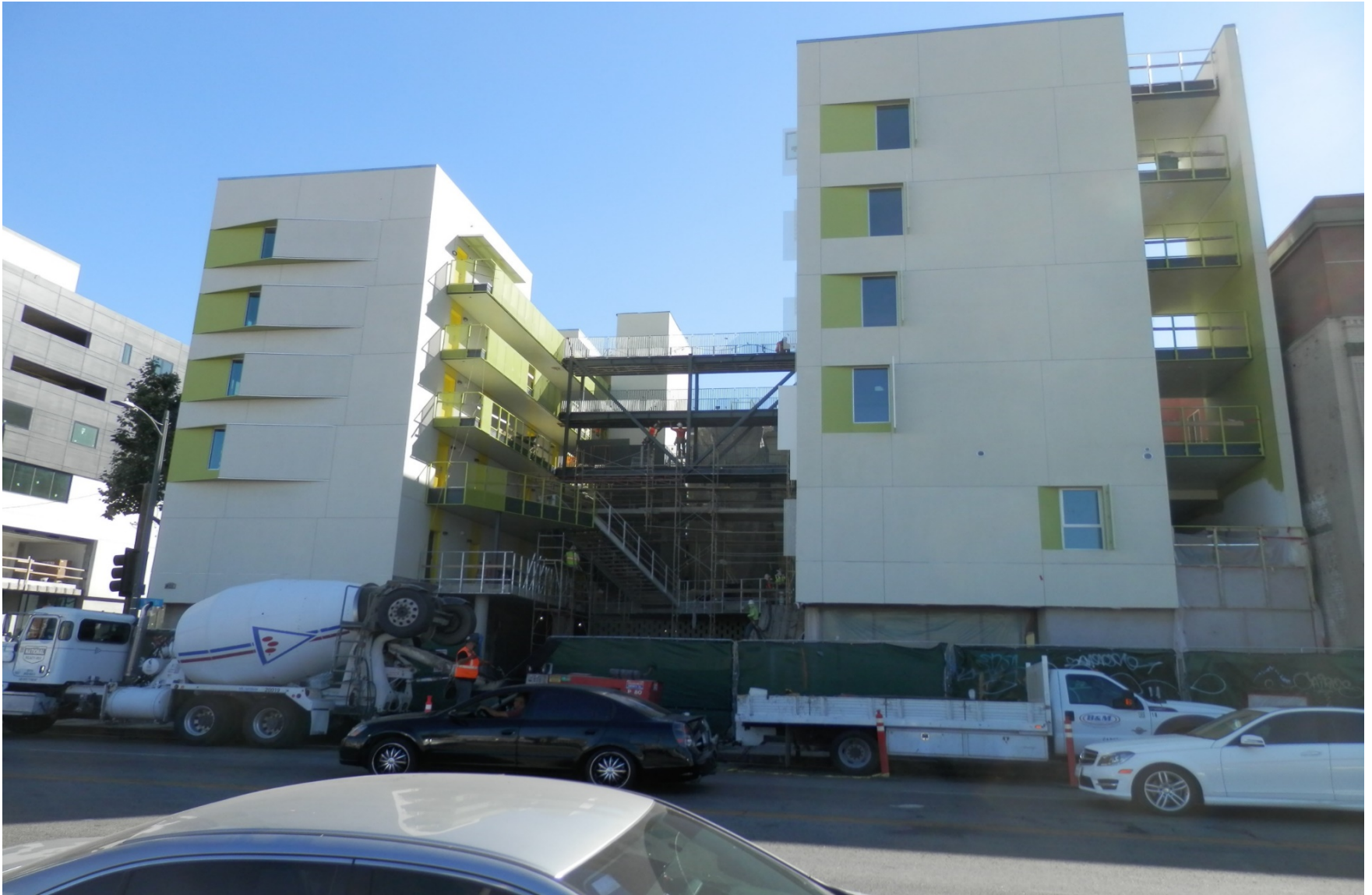
Located at 401 E 7 th St. View from across the street of 401 E. 7 th St.
