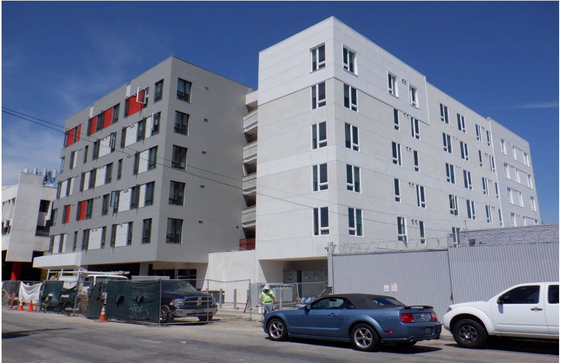
Path Metro Phase 2. View of site at corner of Beverly Blvd & Madison Ave.
